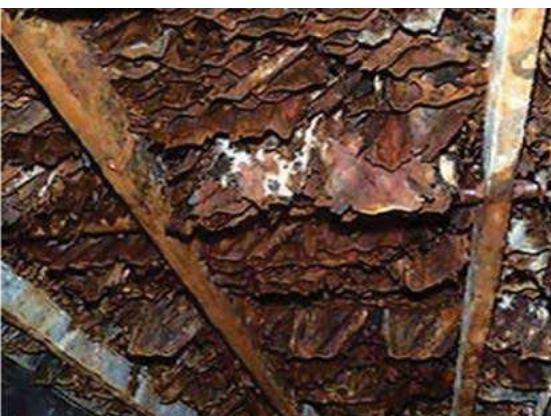
AIR-HEATER CORROSION TYPICAL OF HALIDE USE
