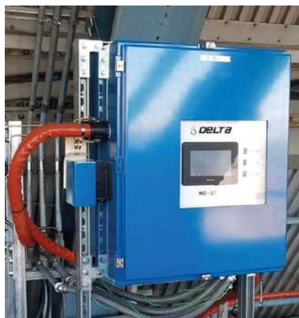
DELTA'S CUSTOM EXTRACTIVE PROBES AND LOCAL INSTRUMENT CABINET
